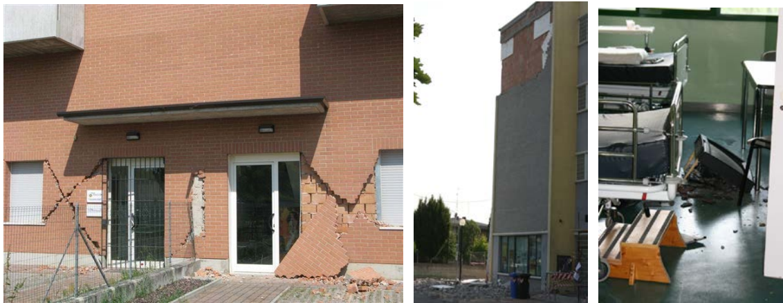
Photographs: External and internal damage examples on Hospital buildings after the Emilia 2012 earthquake (photographs by Masi et al., 2013)
