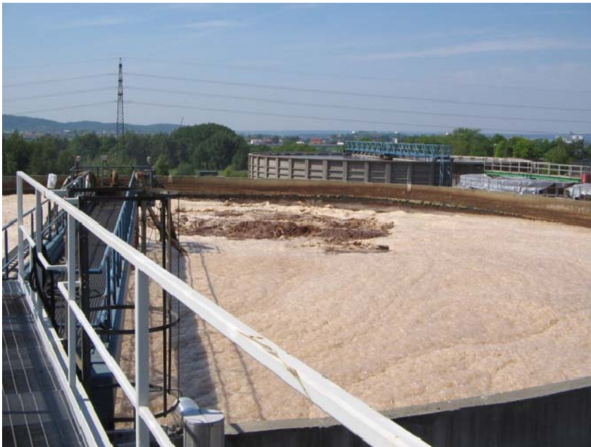
Figure 1.1. One of the aeration ponds at the biological treatment plant at Borregaard Ind. Ltd. (Photo: FFI).
