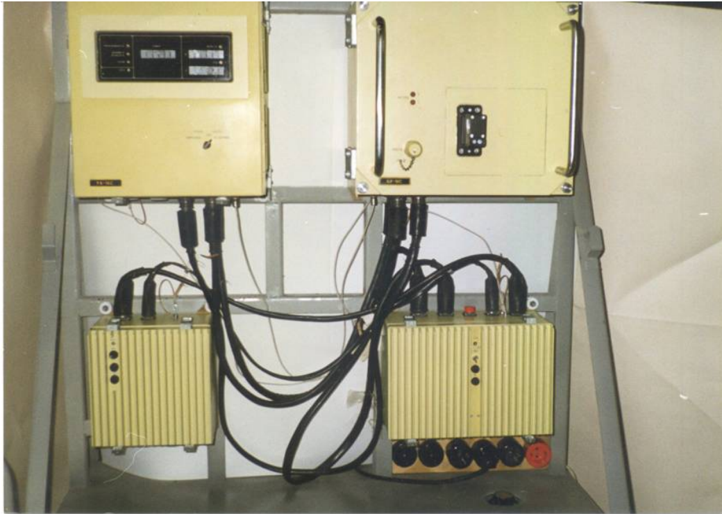
Figure 4. KID-08S TLD reader unit mounted in the Nuclear Radiation Safety Service Building at FSUE 10 SRZ.
