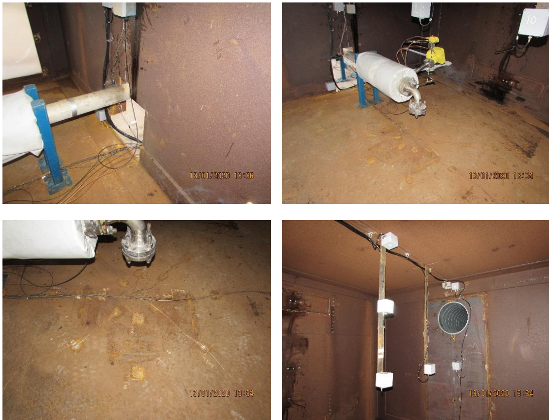
Figure 3.6 Inside the enclosure. Top left photo shows inlet of LH 2 pipe into the closed room. The opening around the inlet was sealed in some of the tests. Top right photo shows the release pipe with release valve and by-pass valve (yellow boxes). The bottom left photo shows the thermocouples on the floor beneath the release point. The bottom right photo shows the vent opening and instrumentation (white boxes) with thermocouples and oxygen sensors. The opening to the vent mast was sealed in some of the tests.
