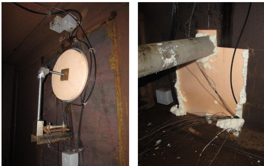
Figure 3.15 Sealing of opening to vent mast to the left. The sealing was connected to a device, which allowed for removal of the sealing from the control room when desired. Additional foam sealing of lower vent opening to the right.
