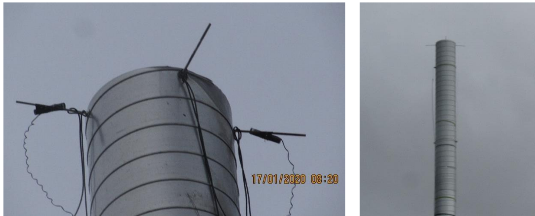
Figure 3.19 Location of ignition devices on top of the vent mast.
